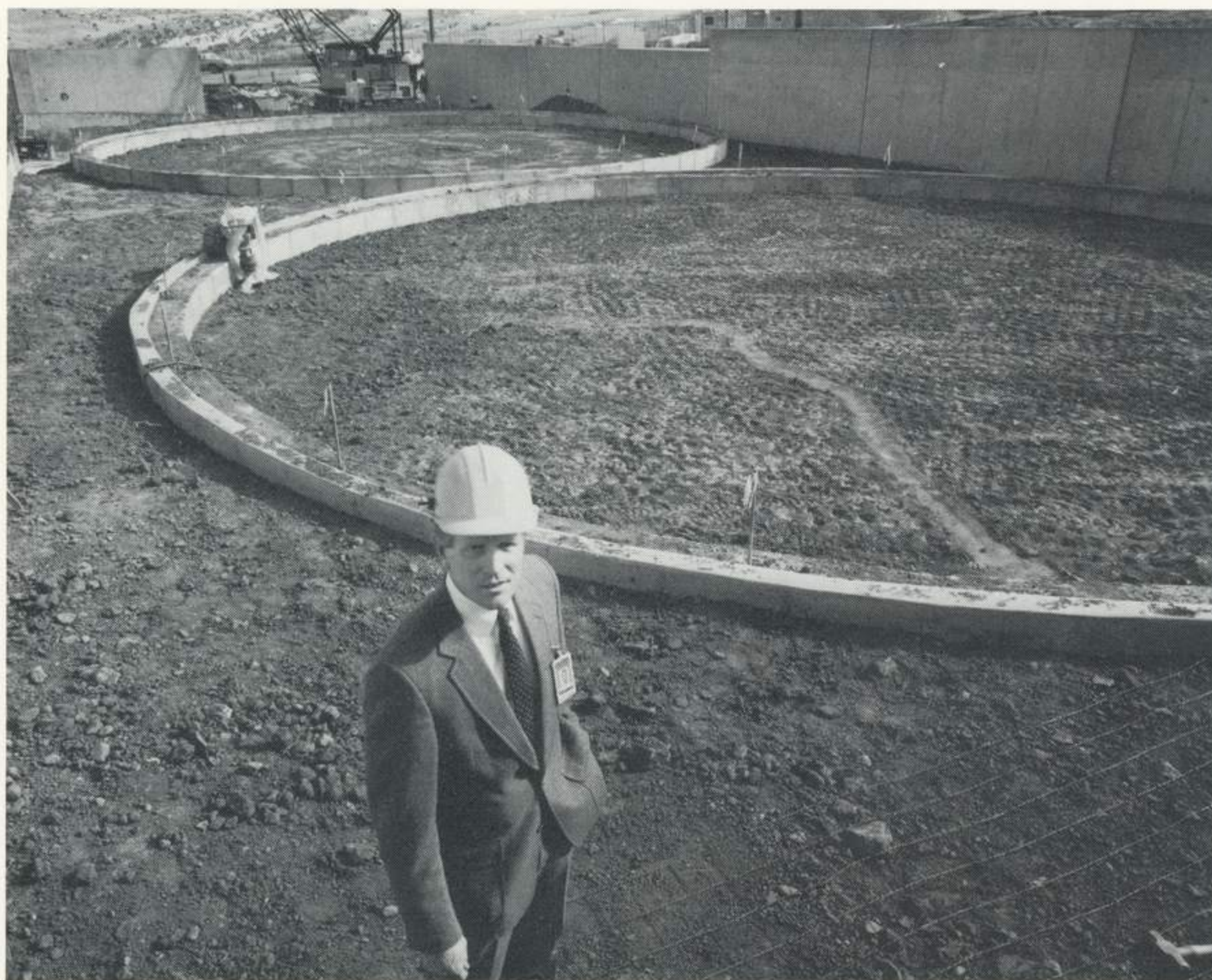
Robert McMullen, director of Environmental Management, stands in the new foundation for a containment area that will consist of three 500,000-gallon tanks, part of a two-phase plan.
