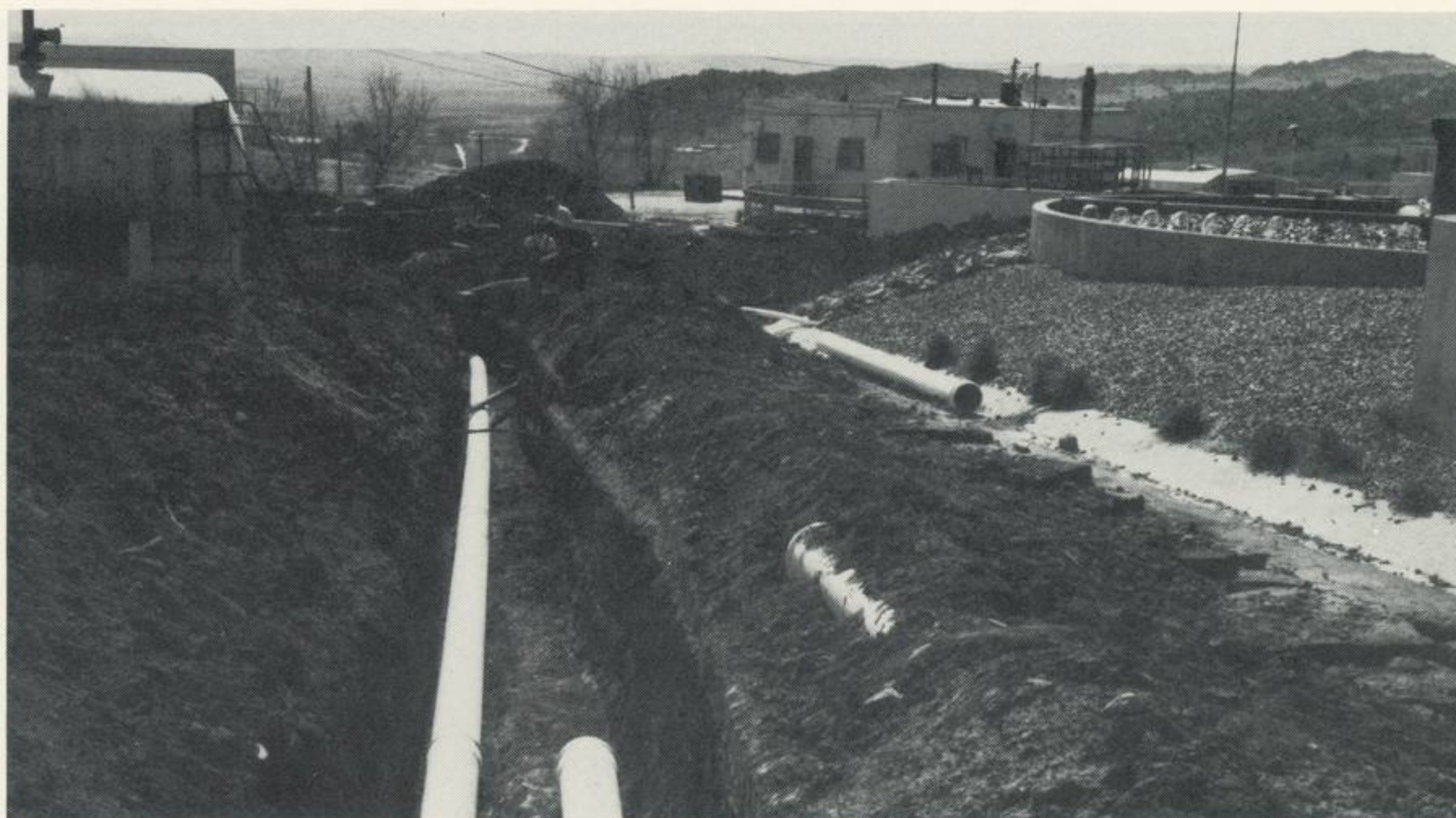
New pipeline was installed at Waterton to replace an alkaline transfer line from chemical milling to the waste treatment plant that broke in March. Future plans call for a double-walled pipeline to be installed above ground. The new pipeline will include sensors to detect any leakage.
