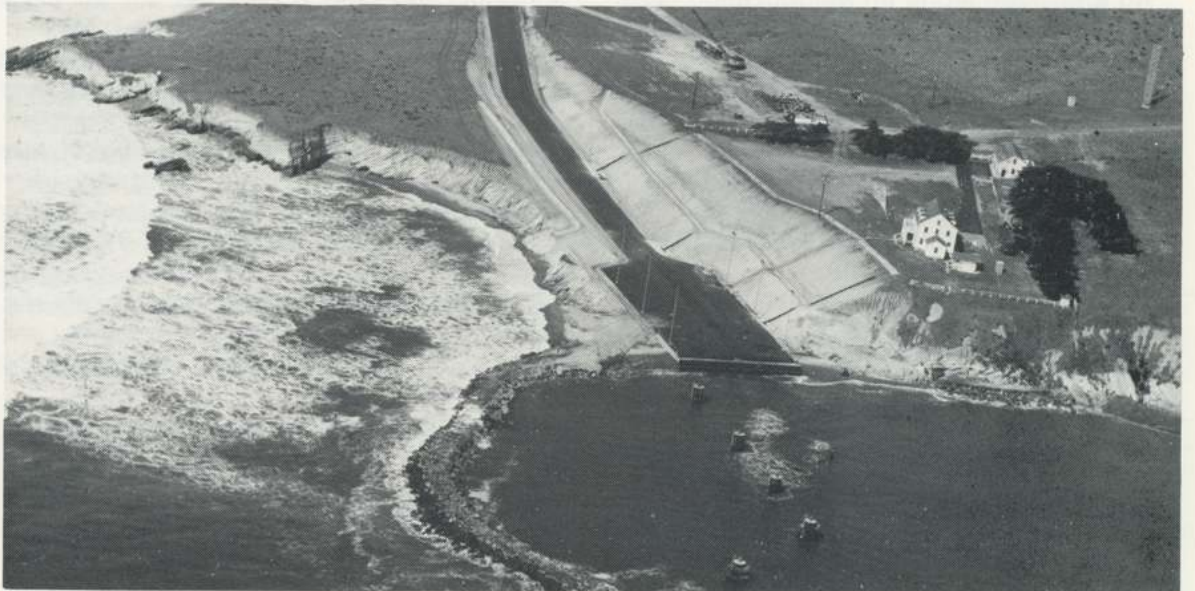
The 2.3-mile external fuel tank tow road and harbor, located at the old Coast Guard boathouse area, south of Point Arguello CA, is nearing completion. Dredging of the harbor is expected to be completed this August. The harbor is the point of entry for the external tank which will arrive at Vandenberg Air Force Base via the Panama Canal from Martin Marietta's Michoud division at New Orleans. The tank will be mounted on a transporter in Louisiana and shipped on a covered barge formerly used to tow Apollo segments to Florida's Kennedy Space Center. The tank on its transporter will be unloaded in California and towed by a large tractor to the external tank checkout facility. Later, it will be towed over the remainder of the route to the launch pad and erected between the two solid rocket motors of the space shuttle.
