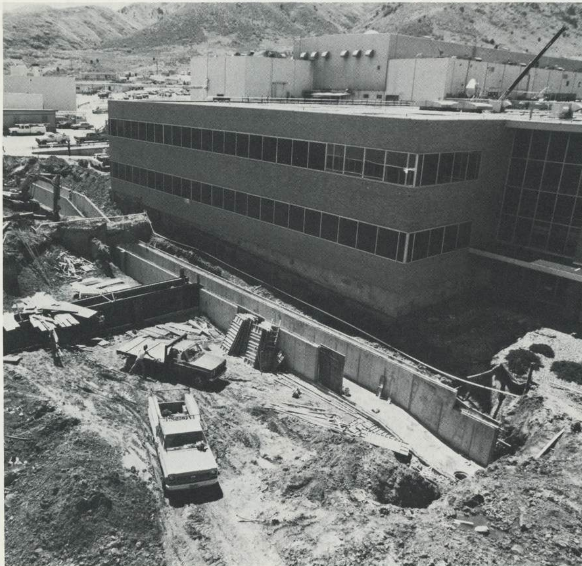
A three-story addition connecting the engineering and administration buildings is nearing completion.
