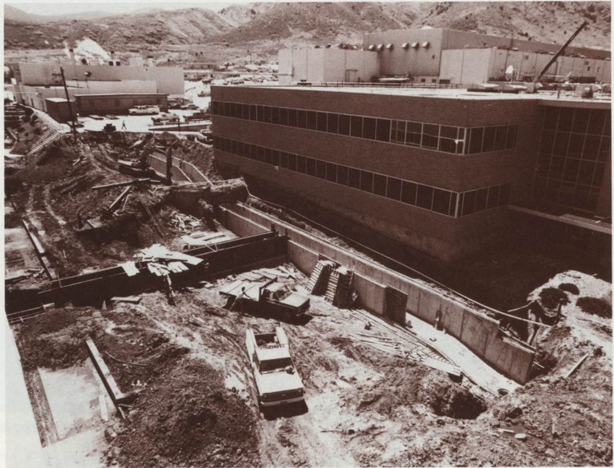
Excavation for addition to the administration and engineering buildings has eliminated direct access between the two buildings. Work on the addition is on schedule, with completion scheduled for January 1983.
