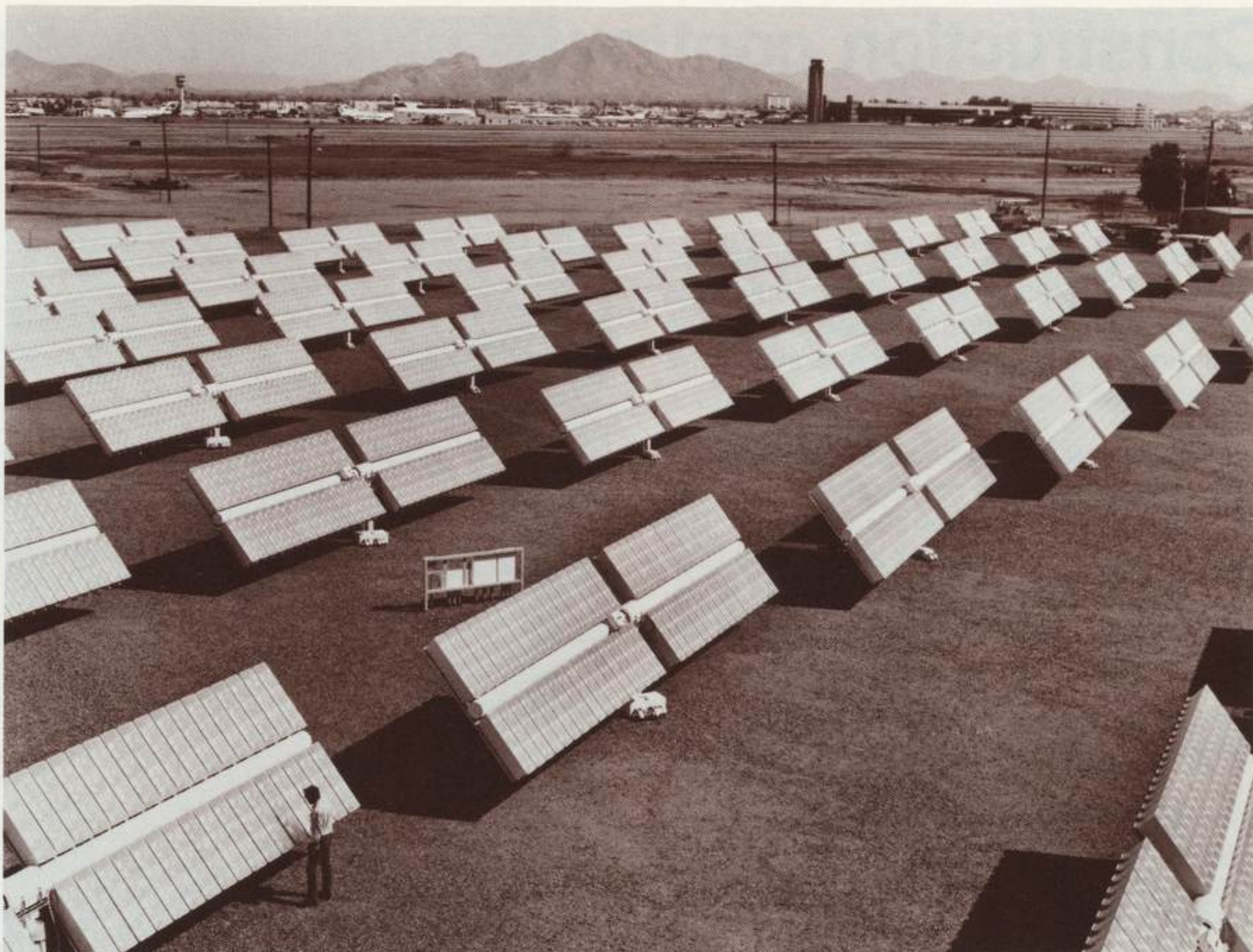
Photovoltaic solar arrays have begun generating electricity at the Sky Harbor International Airport near Phoenix, Arizona.
