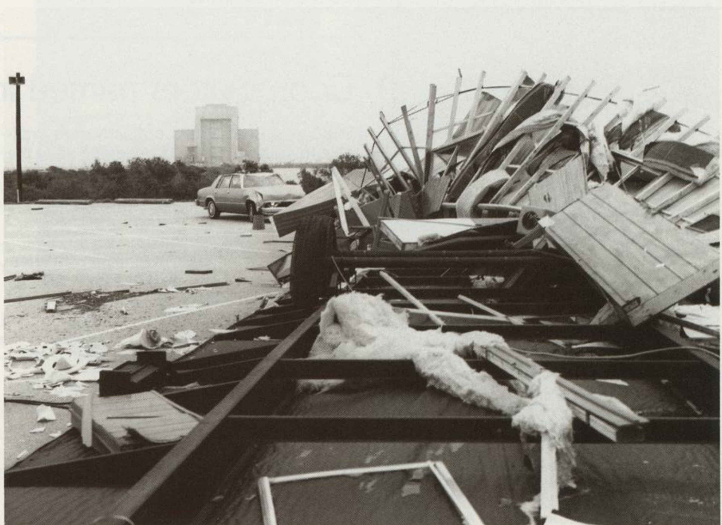
A tornado touched down recently in the Titan III launch area at Cape Canaveral. The upside-down trailer and the leased car near it sustained the only damage. The trailer had been the temporary offices of the Shuttle payload integration facility staff. The twister struck at 4:47 pm, 17 minutes after normal office hours. No one was injured. Building in the background is the solid motor assembly building that will house the Shuttle payload integration facility.
