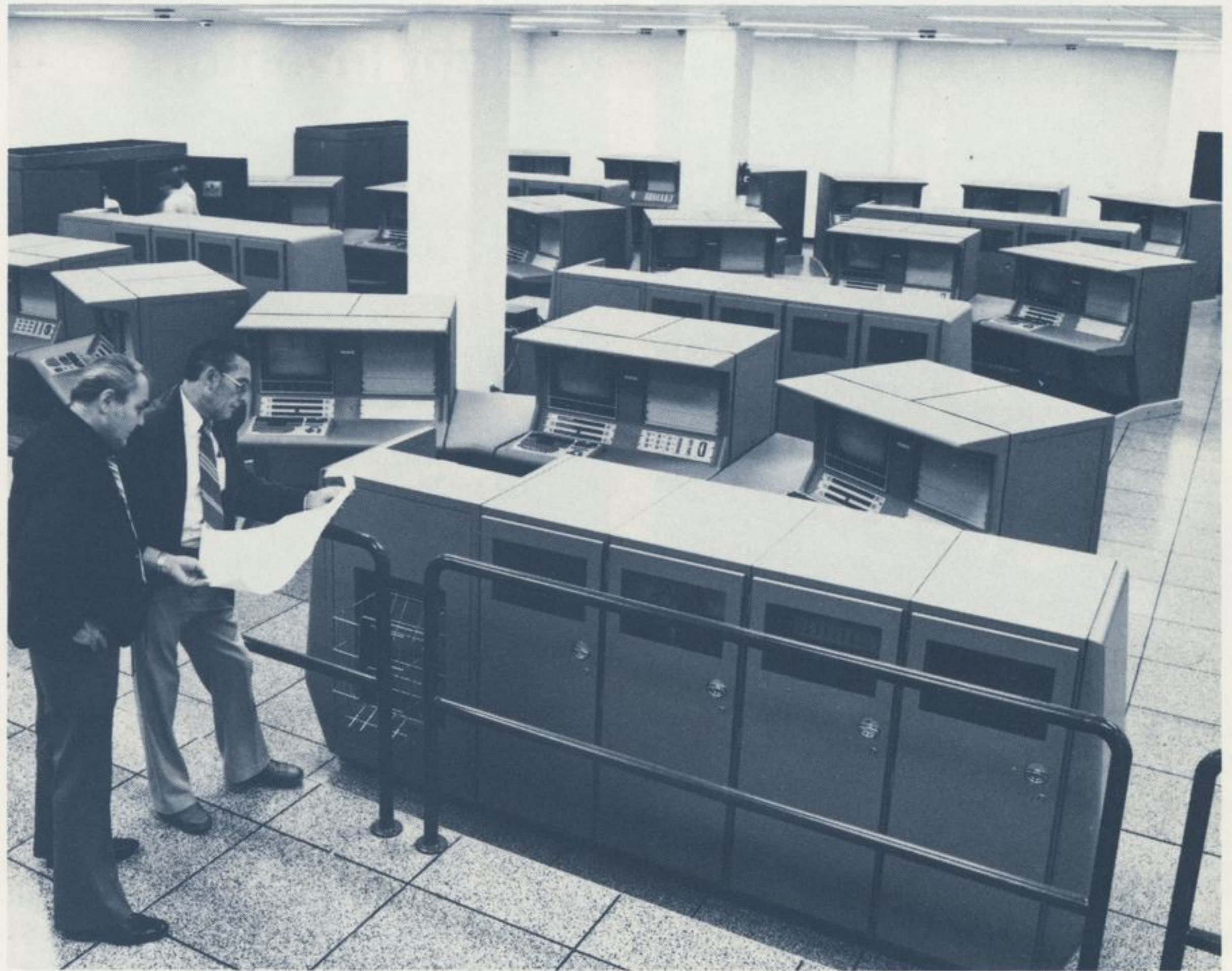
A computer printout from the recently installed CCMS equipment at the Space Shuttle launch control center is reviewed by Vandenberg operations technicians James M. Money and C. Gary Winsell.
