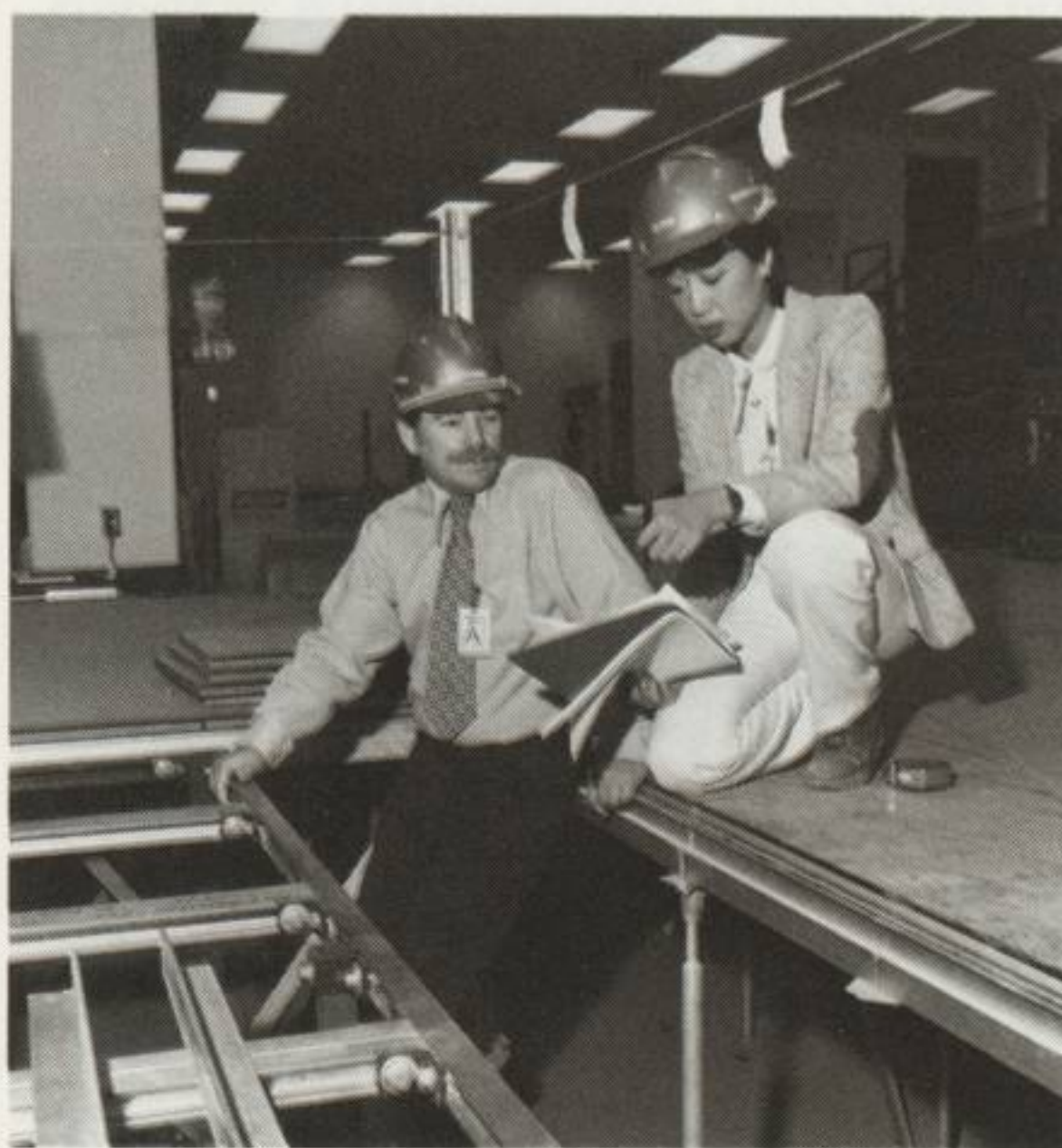
Reviewing installation requirements for Space Shuttle ground support system equipment are, left, Thomas R. Brown, senior installation engineer, and June L. Yee, resident engineer for ground support systems at the launch control center.
