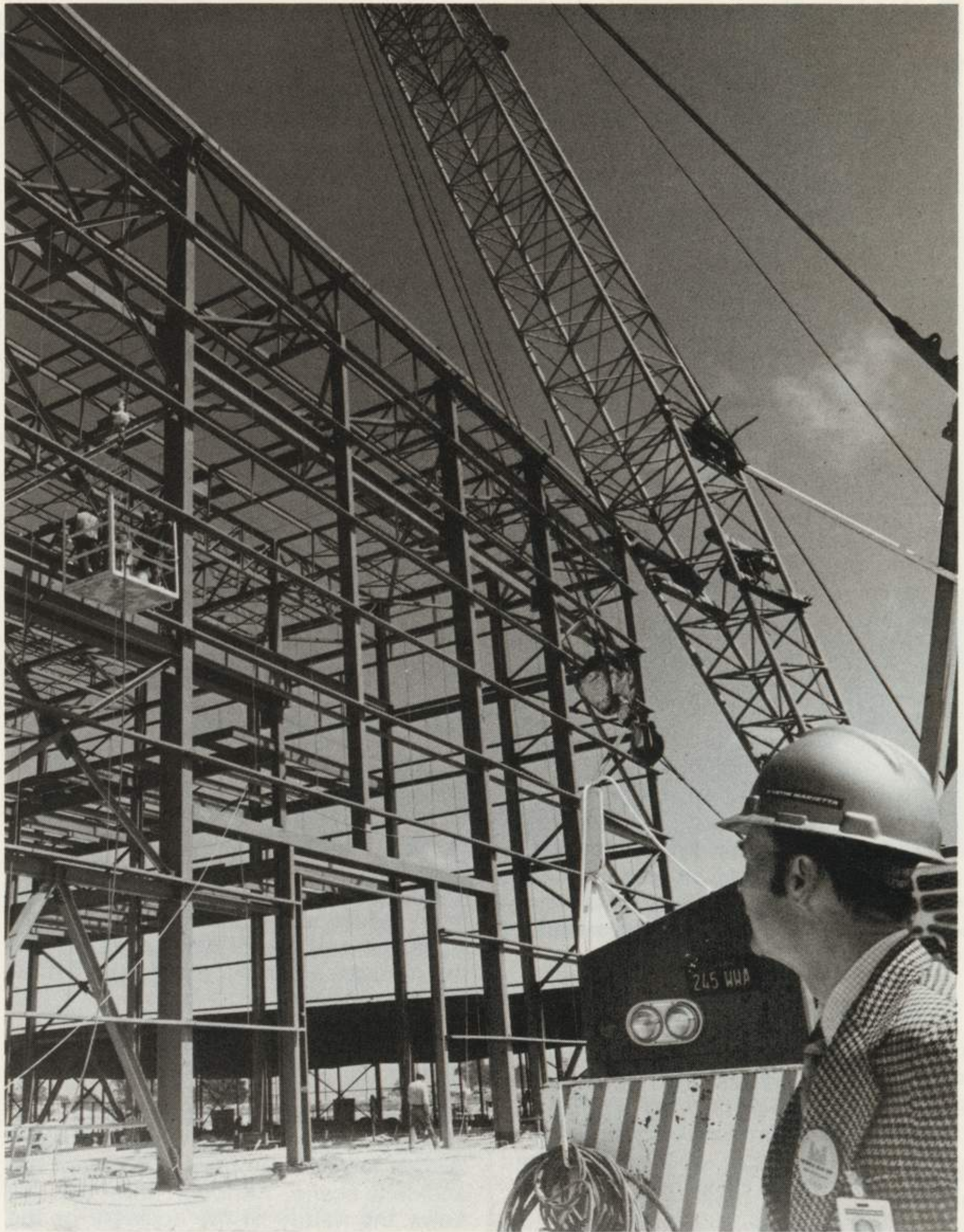
Highbay steel structural work on the Space Shuttle's orbiter maintenance and checkout facility on North Vandenberg Air Force Base is being checked by Paul B. Cusick, senior field engineer for construction surveillance at Vandenberg operations. The foundation work, which included the 50-foot deep payload deservicing pit, was completed in November 1980. The facility will provide for gaseous nitrogen, helium, oxygen, and hydrogen servicing; hydraulics and fuel cell coolant loop servicing; environmental control and life support system water and freon servicing; installation of payloads and deservicing of returned payloads; and thermal protection system maintenance. Work on the facility will be completed in early 1982.
