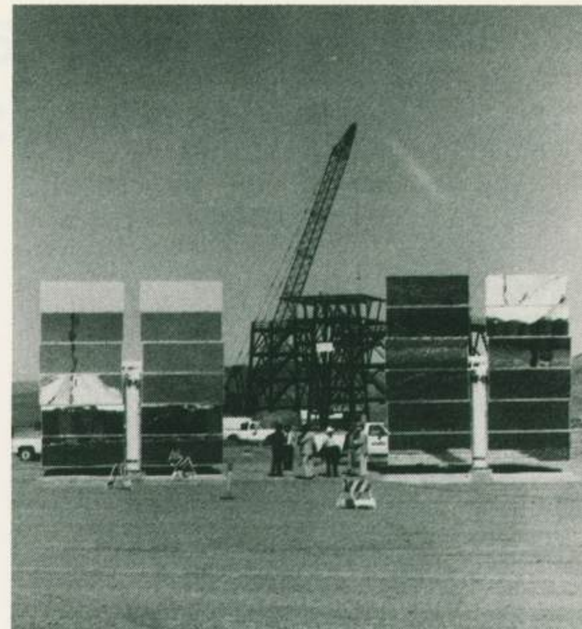
Denver-produced heliostats at the Barstow Solar One facility flank central receiver construction.
