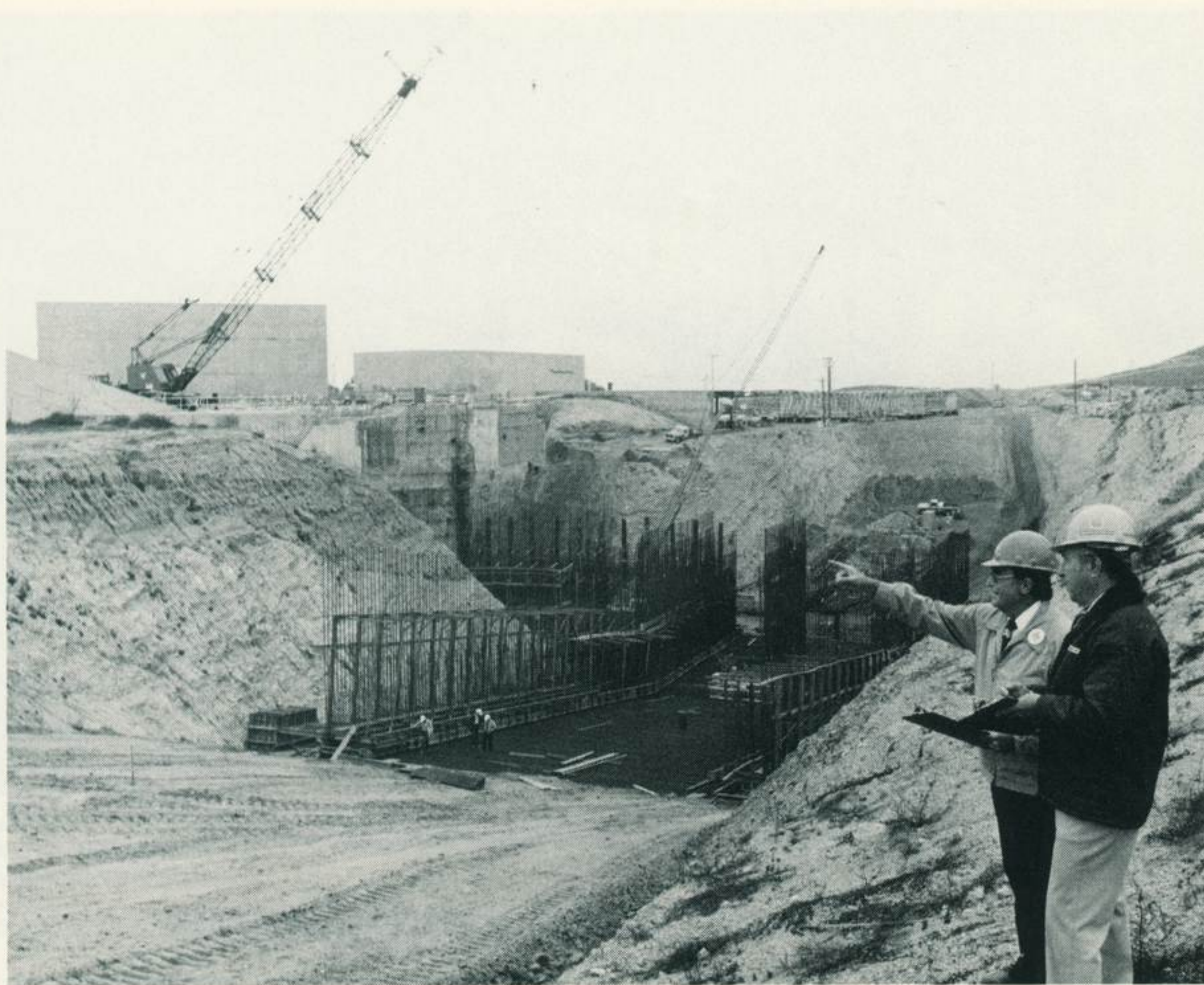
Vernon L. Dunn, Denver Aerospace manager for DOD/STS ground support systems facilities, right, and Roy Graffham, The Ralph M. Parsons Company GSS construction surveillance manager, check construction progress of solid rocket booster and main engine exhaust ducts. The Space Shuttle launch pad is under construction at Vandenberg Air Force Base.
