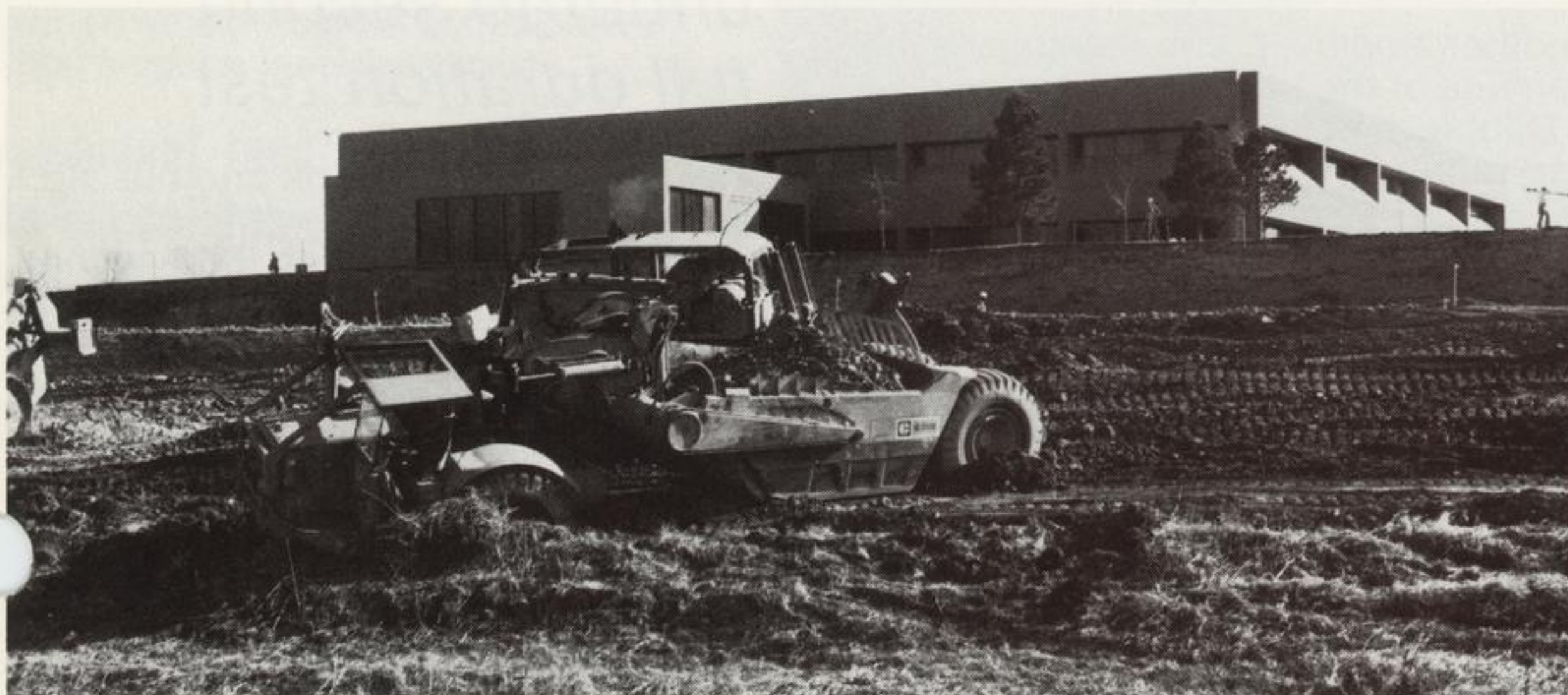
Earth-moving equipment is at work at the site of the four-story addition to the division's office building at Hampden and Wadsworth. The addition is to be completed in early 1981.
