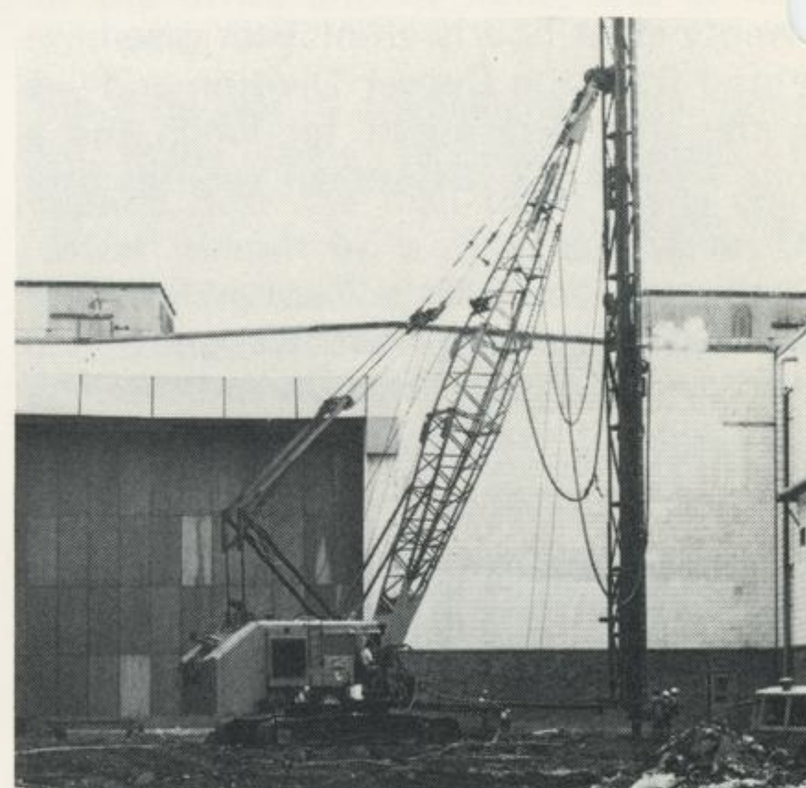
Boh Brothers Construction Co. is working on foundation and utilities for addition.
