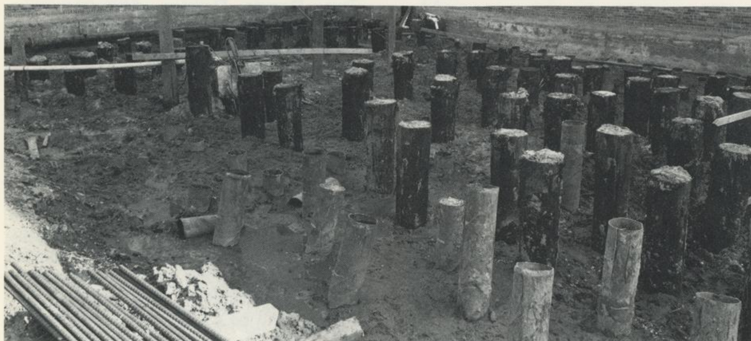
More than 500 wooden pilings were driven 60 feet into Louisiana silt to support the 100-foot tall addition to the high bay building at Michoud.
