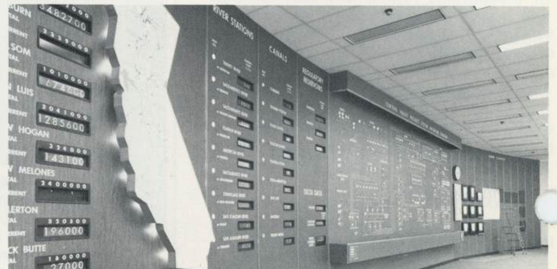
Display panel at Sacramento Central Valley Project control center keeps operators continually informed of facilities status throughout area.
