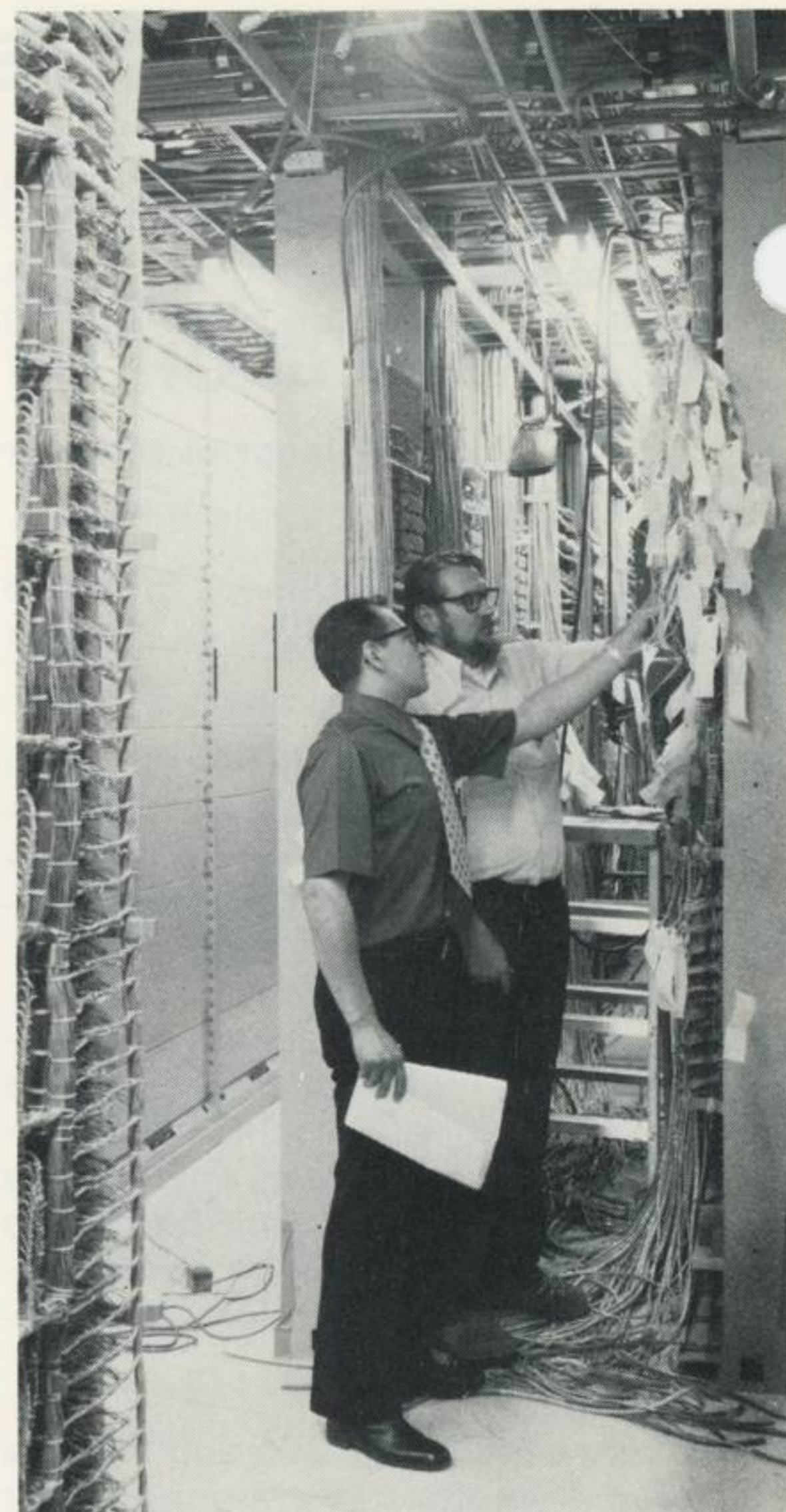
Virgil Jaramillo, who is coordinating Centrix installation for the division, discusses wiring for the system with Western Electric installer Richard T. Dowe.
