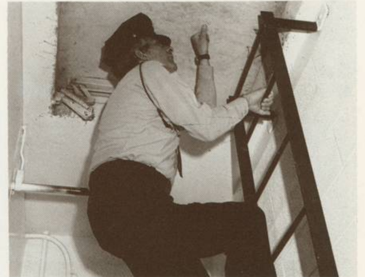
Equipment function is checked.
